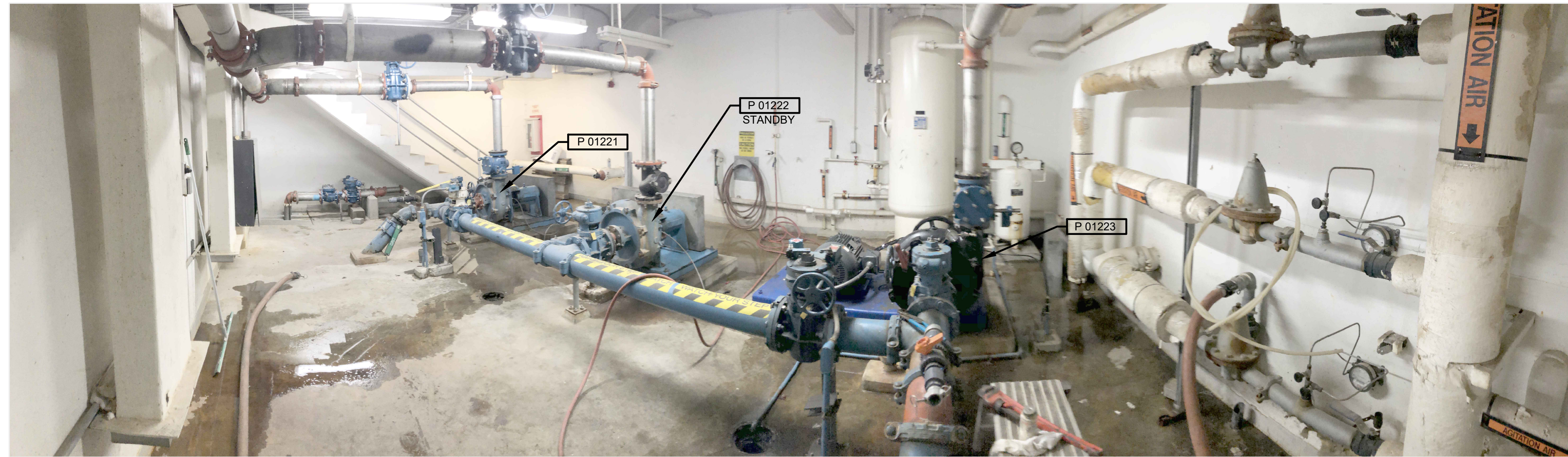
P2 PHOTO GRIT PUMP ROOM
